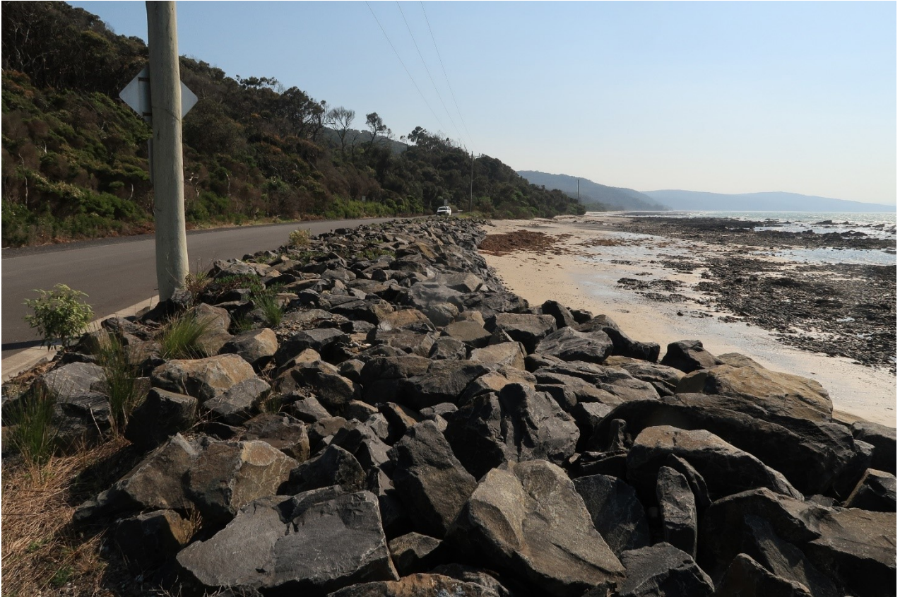
Figure 6 An example of rock walling, Central Management Unit, Walkerville Foreshore Reserve, October 2023
